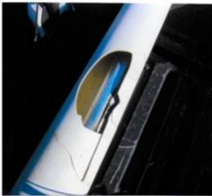
The old setups allowed rain to enter the mounting poles, which froze and split the pole, destroying the predator guards. Photos taken by Allen Jackson.
